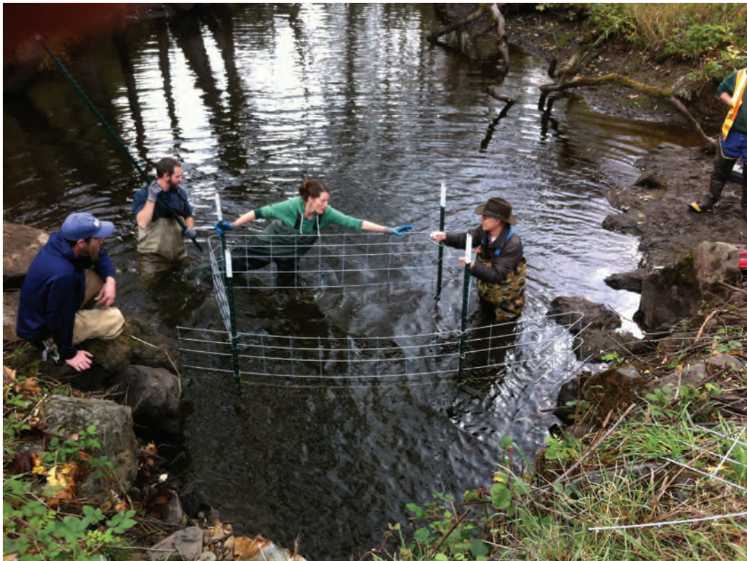
Figure 50. Installing a “beaver deceiver” pipe through a beaver dam downstream of the SR 116 culvert to control the water level at the culvert (top) and a trapezoidal fence upstream of the culvert to prevent beaver from plugging it (bottom).
