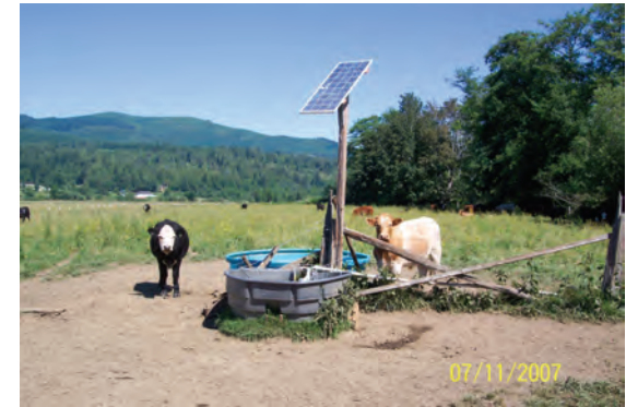
Solar pump water supply system
