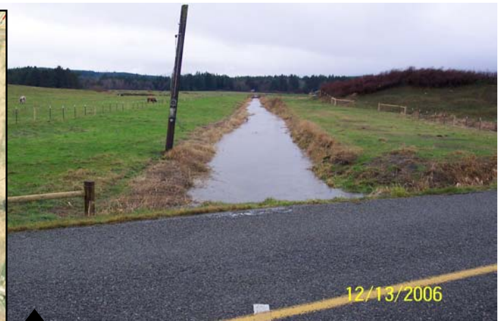
▲ In summer 2006, aquatic vegetation was removed from the stream channel, LWD was added to the channel, 2,900 feet of riparian fencing was installed, and a livestock bridge was rebuilt. A stock watering trough and a heavy use area was installed in the fall of 2008 completing the project
